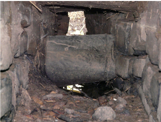
Blocked road culvert at Helland
