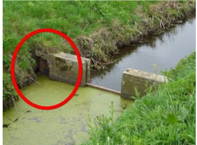
Washed out headwall Back Ditch structure – due for replacement 2010
